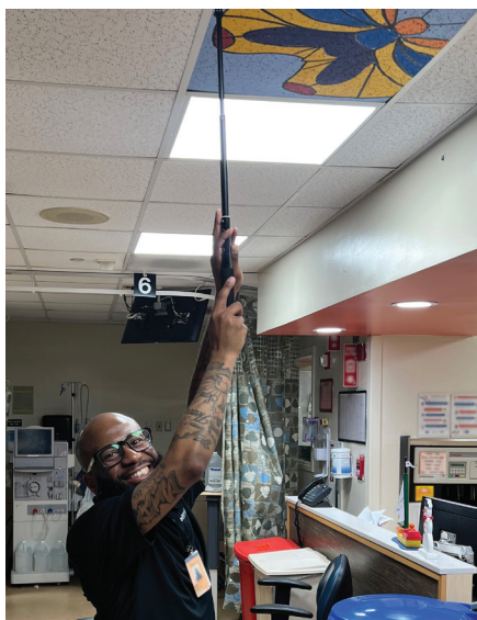
Ergotron's Ted Hightower installs beacons for RhythmConnect at Montefiore Einstein
